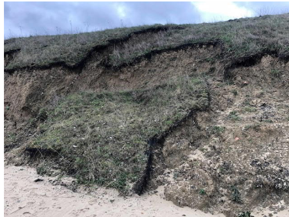
Fig 3.1E. Cliff condition at beach level.
