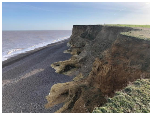
Fig 3.3D. Cliff face condition from top of cliff.
