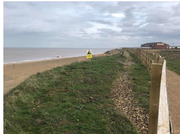
Fig 3.1B. Embankment fenced off due to erosion.
