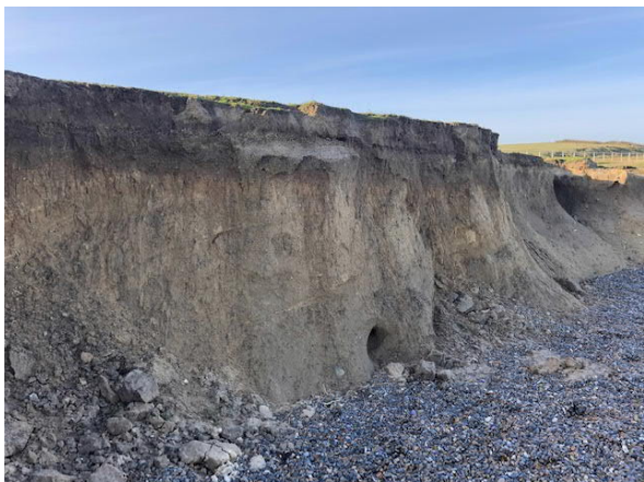
Fig 3.4E. Cliff face condition.
