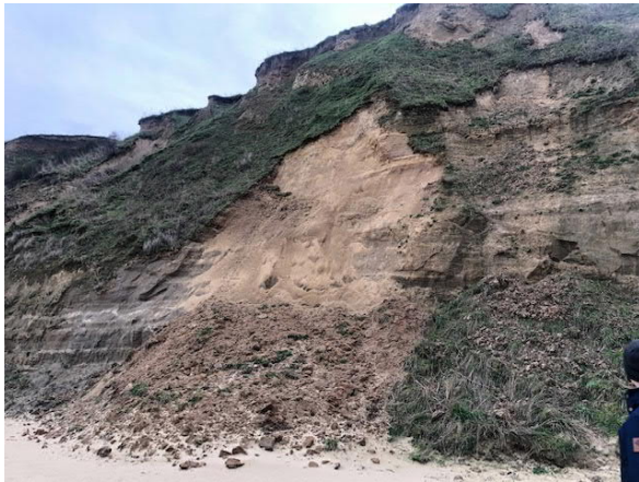
Fig 3.2E. Cliff condition at beach level.
